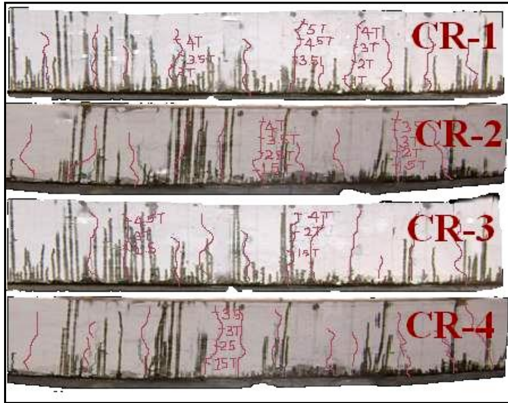
Figure 6 Crack pattern of perfect and corrosion control beams
