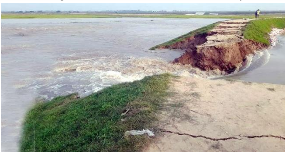
Image 4 An embankment collapses in Sunamganj Dharmapasha Haor inundating Boro crops (adapted from TBS, 2022a).
